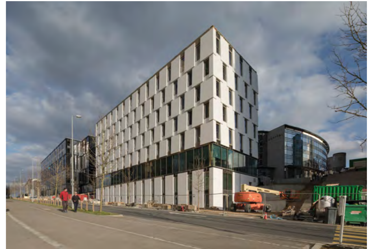
L'hôtel Mama Shelter et le commissariat de police Mama Shelter Hotel and the police station
