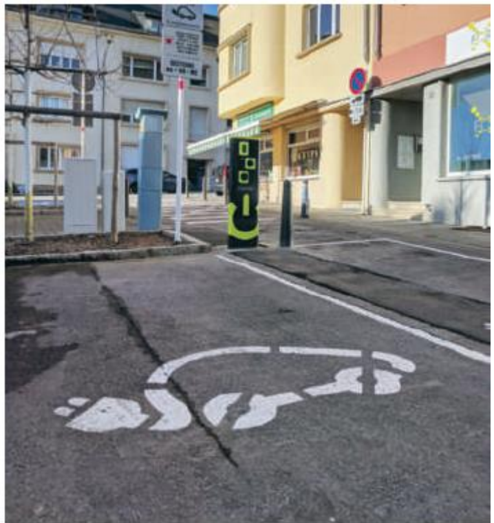
Parking space with a “Chargy” charging station (MDDI)
